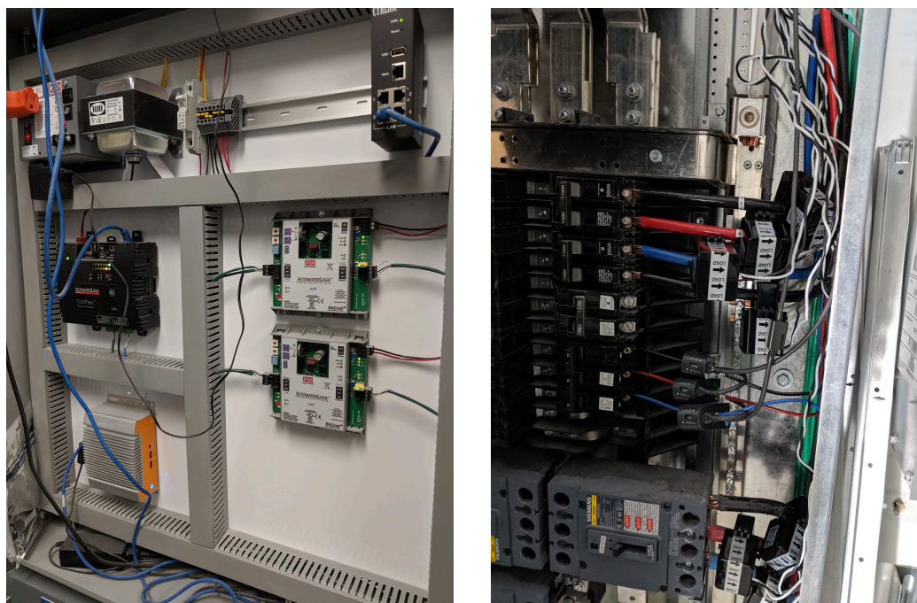
Existing BMS (left) and example of sensors installed in panels at ARM SJ (right)
